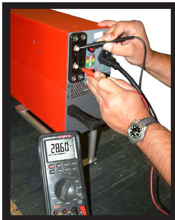
Figure 8-12: Test DC Receptacles 8-7
